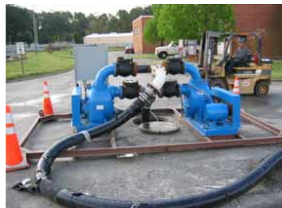
A typical large-capacity bypass pumping system working from an existing manhole. Picture courtesy of Hampton Roads Sanitation District, Virginia, USA.
