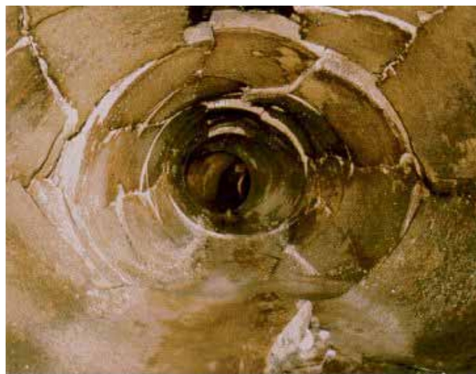
Multiple fractures in a clayware pipe – this is representative of the most severe damage that can be renovated using cured-in-place lining techniques
