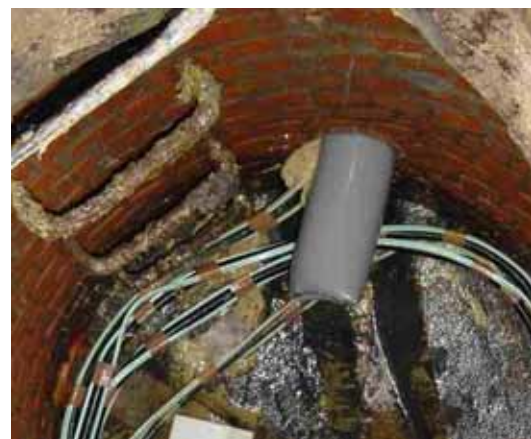
‘Inversion Lining’ technology being used to install fibre optic cabling in a lateral sewer connection for a residential or business feed.
