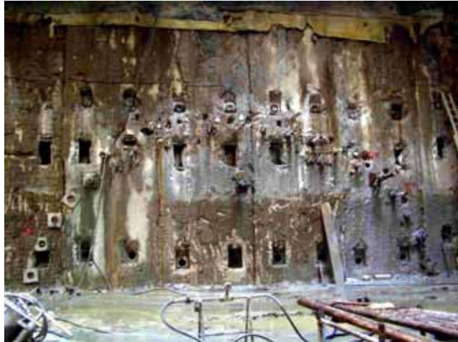
An arch of borehole installed using HDD technology as part of a ground stabilisation programme prior to a major tunnel installation.
