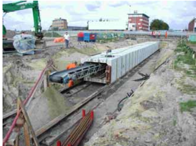
Installing a box section under a railway embankment. In this instance using pulling rods to apply the ‘jacking’ force as opposed to rear positioned hydraulic jacks.
