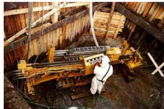
Using HDD to install ground remediation drainage pipelines. Note the personnel protection used for the crew. Picture courtesy of Mining Communications Ltd.
